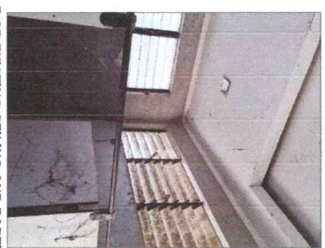
MALE CR EXISTING CEILING AND PARTITION NOTE: CHANGE CEILING PLAN, LIGHTINGS INTO SURFACE TYPE PIN LIGHT & PROVIDE EXHAUST FAN, INSTALL NEW COMPACT LAMINATED BOARD PARTITION
